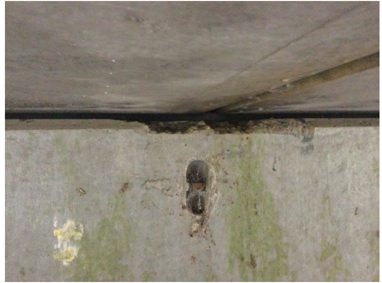
Small spall on left bank cap
